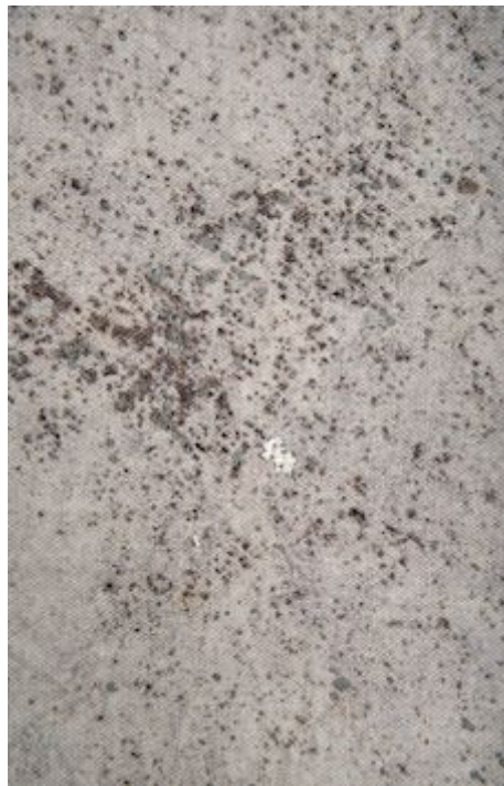
Another example of transferred paint from the floor
